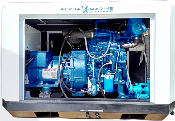
Alpha Marine Generator
